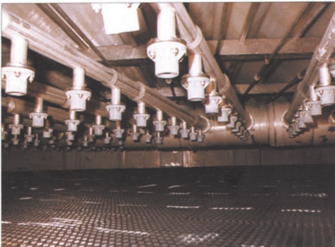
View in the absorber zone of a flue-gas desulphurization plant
