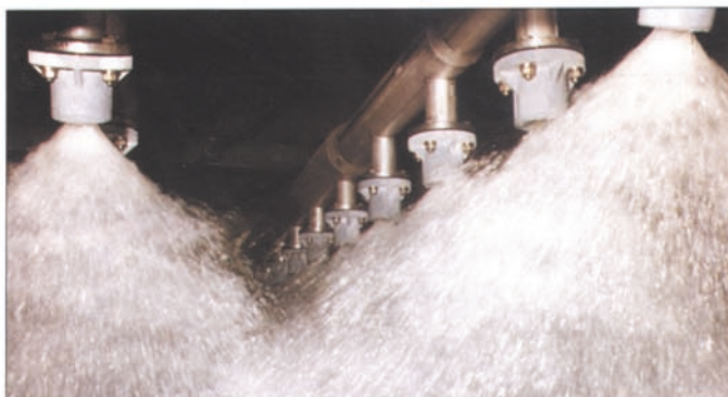
Full-cone nozzles in a flue-gas desulphurization plant
